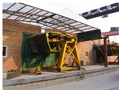
Figure 11: Segment Curing Chamber
